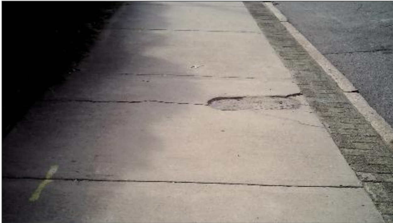
Utility Obstruction in Pavement
