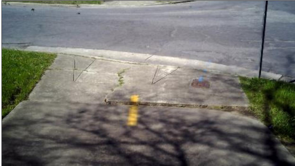
Sinking in Pavement
