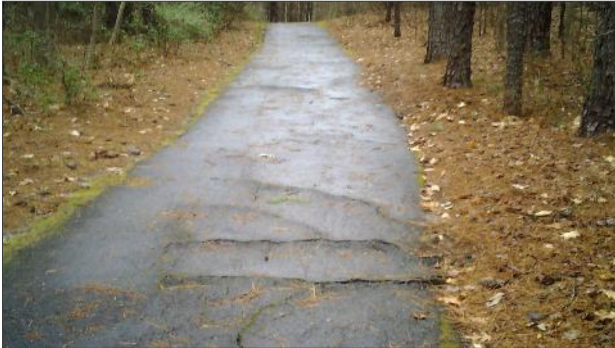
Cracking in Pavement
