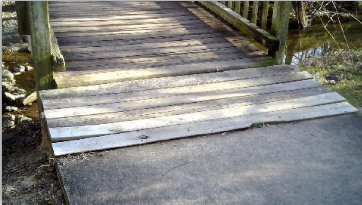
Missing flush transition
