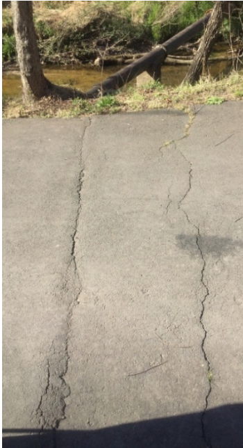
Minor Pavement Cracking
